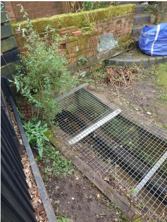
Cover re-instated following forming of working space and excavation and removal of material.
