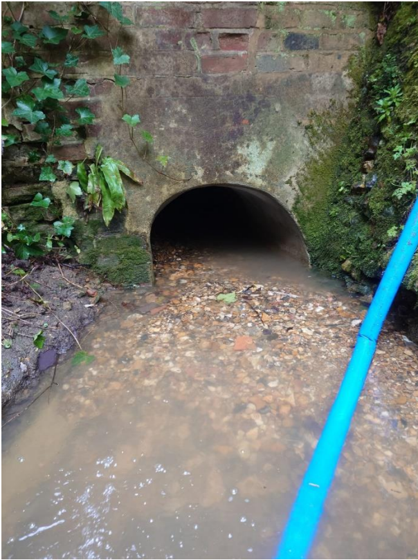
Sediment build up to upstream end prior to commencement.
