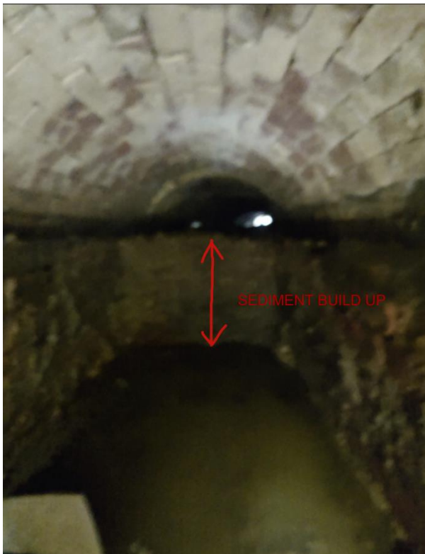
5m into culvert from upstream end showing sediment build up.
