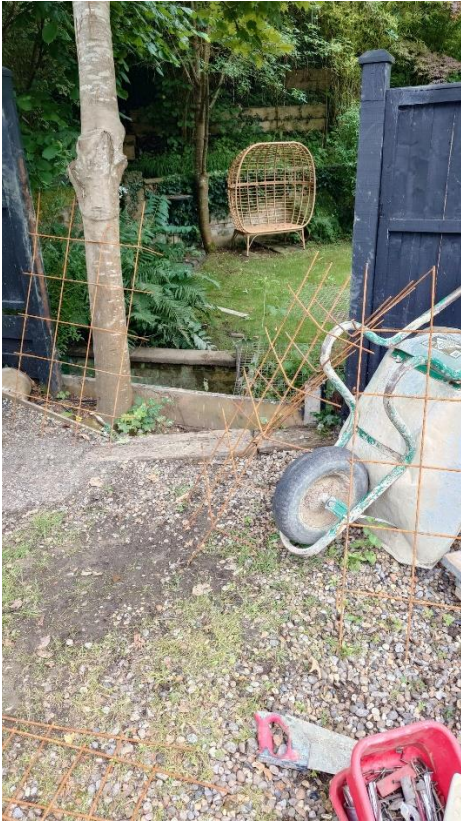
Steel reinforcement prepared for culvert floor and concrete walls to area below driveway
