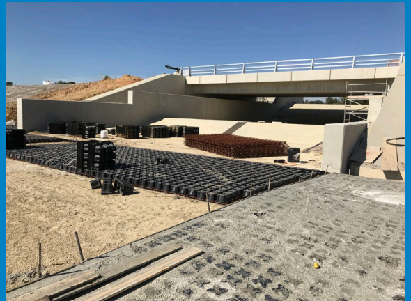
Scour protection being installed at the spillway from the Albury Tributary reservoir
