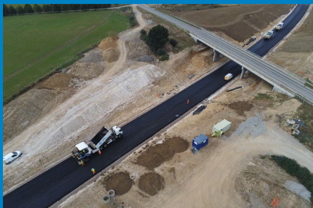
Albury Road and Bridge from above as asphalt is laid across the site
